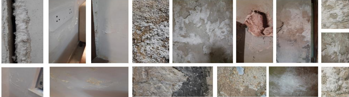
Figure 18 Onsite photos of different locations with mold growth.
